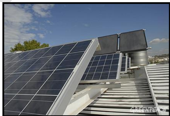
Figure 3.3.1: Solar PV panels atop a roof in Spain
