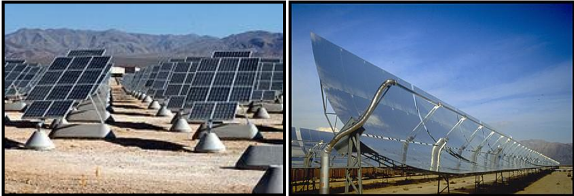
Figure 3.1.6: (a) The Nellis Solar PV Plant in Nevada, USA (b) A CSP Parabolic Trough Solar Farm
